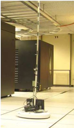
Figure 1: The data center management robot.
